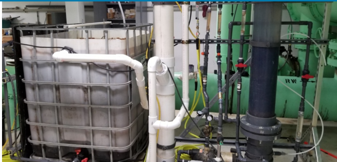
■ ABOVE, THE PILOT project system is set up to test if naturally occurring organisms in New Ulm's groundwater can remove undesired elements without the use of chemicals.
