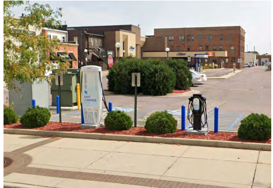
EV charging stations located at the City's parking lot along 2nd St N.
